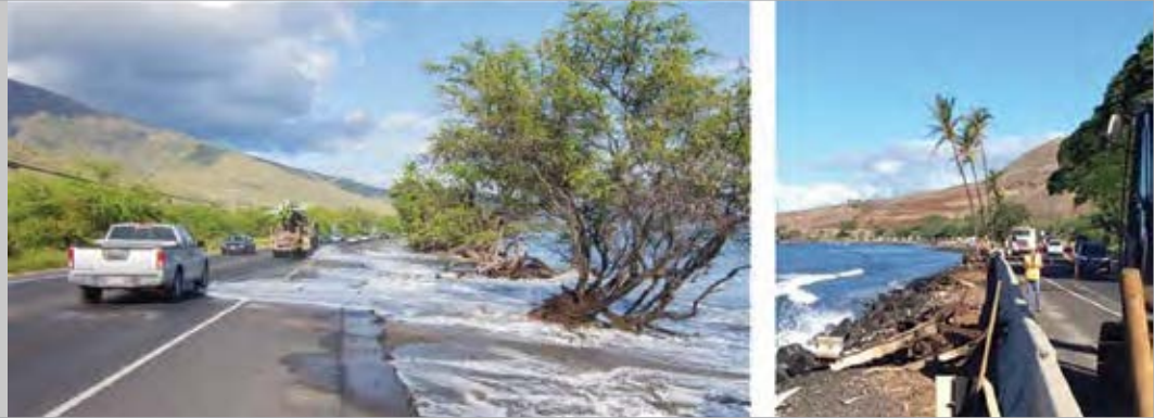
Figure 3.5-2 Honoapiilani Highway Erosion Source: Maui Planning Department
